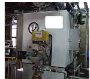
Fujisawa Plant's vacuum dewater drying device
