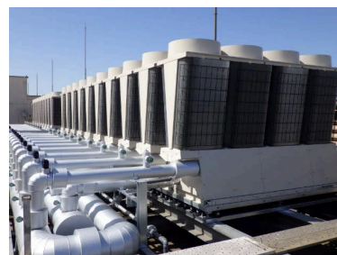
Air-cooled chillers installed at the Saitama Plant
