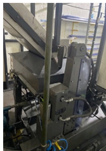
Briquetting equipment installed at the Peterlee Plant
