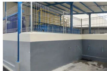
Wastewater treatment facility at AKS Precision Ball Indonesia
