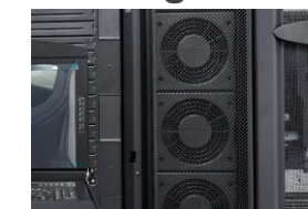
Server cooling fans
