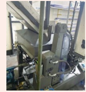
Briquetting facility at the Peterlee plant (UK)
