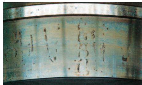
Rust and corrosion
