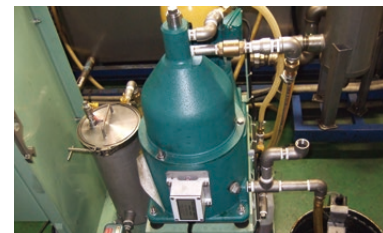
Centrifuge that separates oil and sludge from waste liquid
