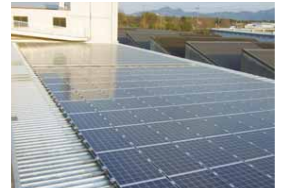
Solar power generating system installed at the Mihara Plant of Inoue Jikuu Kogyo
