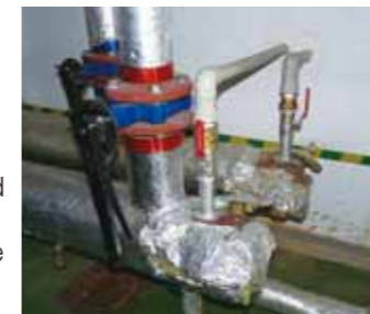
Recovered heat from the air compressor is channeled into the plant's heated water equipment.
