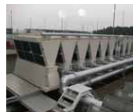
Heat pump at the Fukushima Plant
