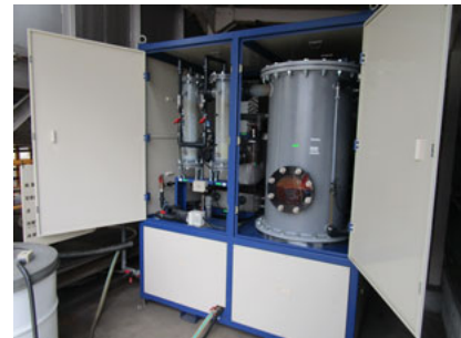
The waste liquid distillation concentrator deployed to Amatsuji Steel Ball Mfg. Co., Ltd. (Shiga plant)
