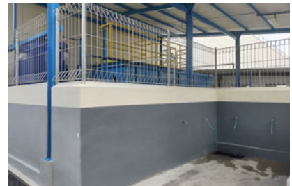
Waste water treatment facility at AKS Precision Ball Indonesia
