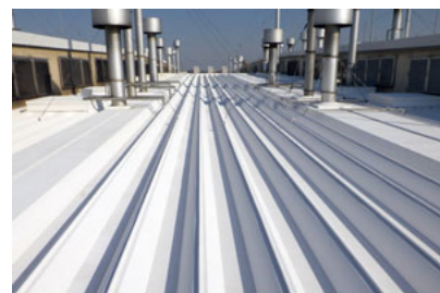
Thermal insulation paint on the roof of the Saitama Plant
