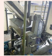
Briquetting facility at the Peterlee plant (UK)
